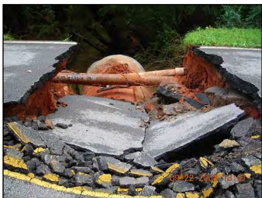
Damaged Water Pipes on Brown Lee Road in Gwinnett County, GA during the September 2009 Flood.
