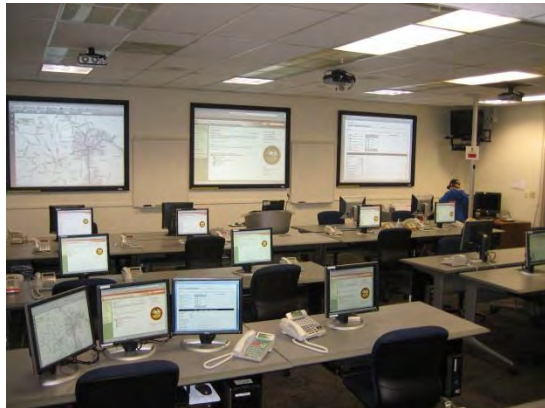
Santa Rosa Emergency Operations Center. Credit: Sonoma County Fire and Emergency Services. Source: Helgren, 2014.
