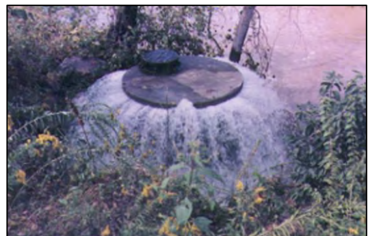
Sewer System Overflow in Johnson County. Credit: Johnson County Wastewater Source: Witt, 2013
