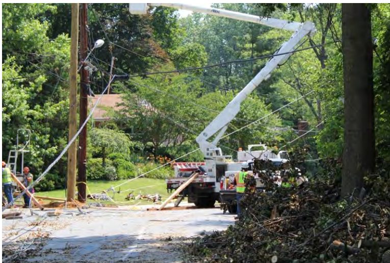
Utilities Work to Restore Power in Montgomery County Following the 2012 Derecho Windstorm.
